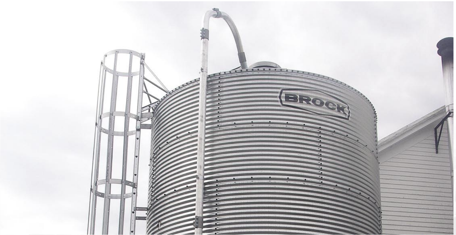
A 36 ton silo located outdoors, adjacent to the boiler room, stores wood pellets. The pellets are automatically delivered to the boiler through an auger system.
