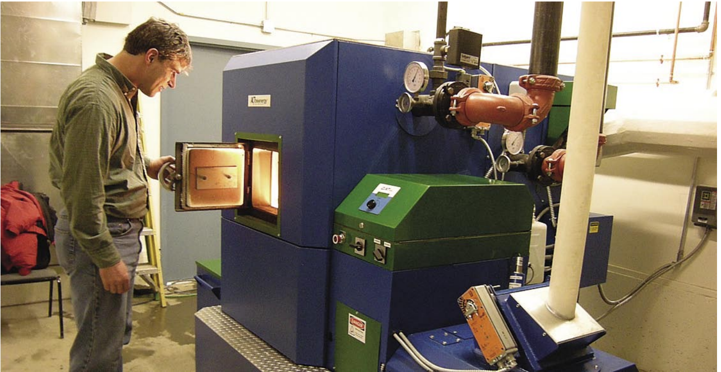
A wood pellet biomass boiler plant was installed to lessen the Academy's dependency on fossil fuel and address facility heating needs.
